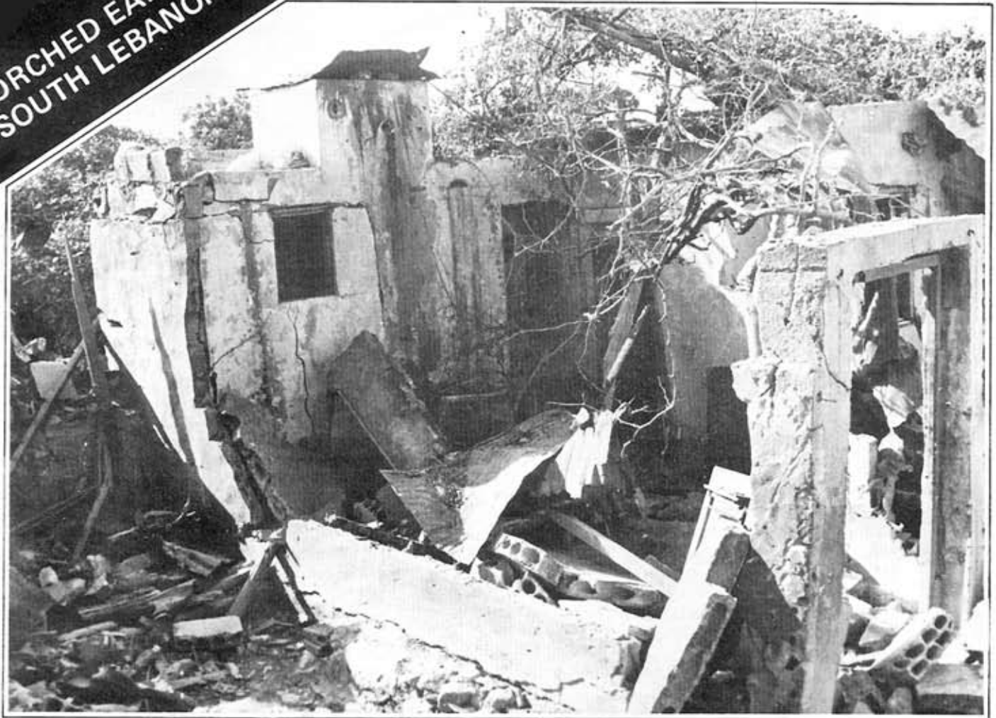
Destroyed huts at Ain Hilweh refugee camp, August 28, 1979
